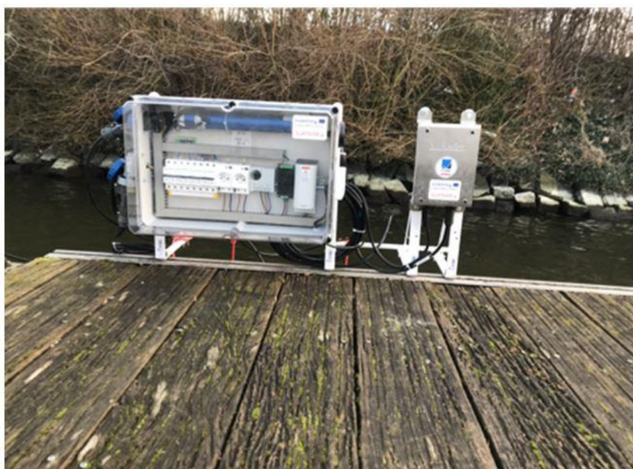
Figure 5 The sensor box installed in zelzate marina in the framework of Socorro project.
